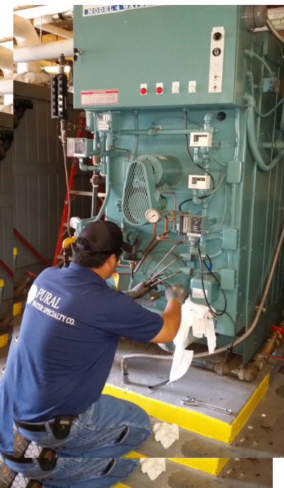
Technician Chad B. doing final inspection before firing up a Steam Boiler at a Hospital.
